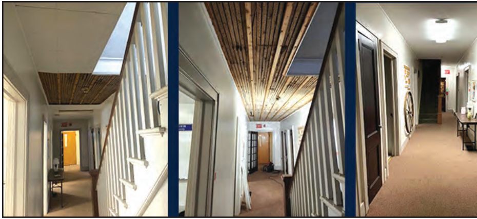
Replacement of lighting, ceiling and drywall was recently done at Carnwath Farms Historic Site in Wappinger.
